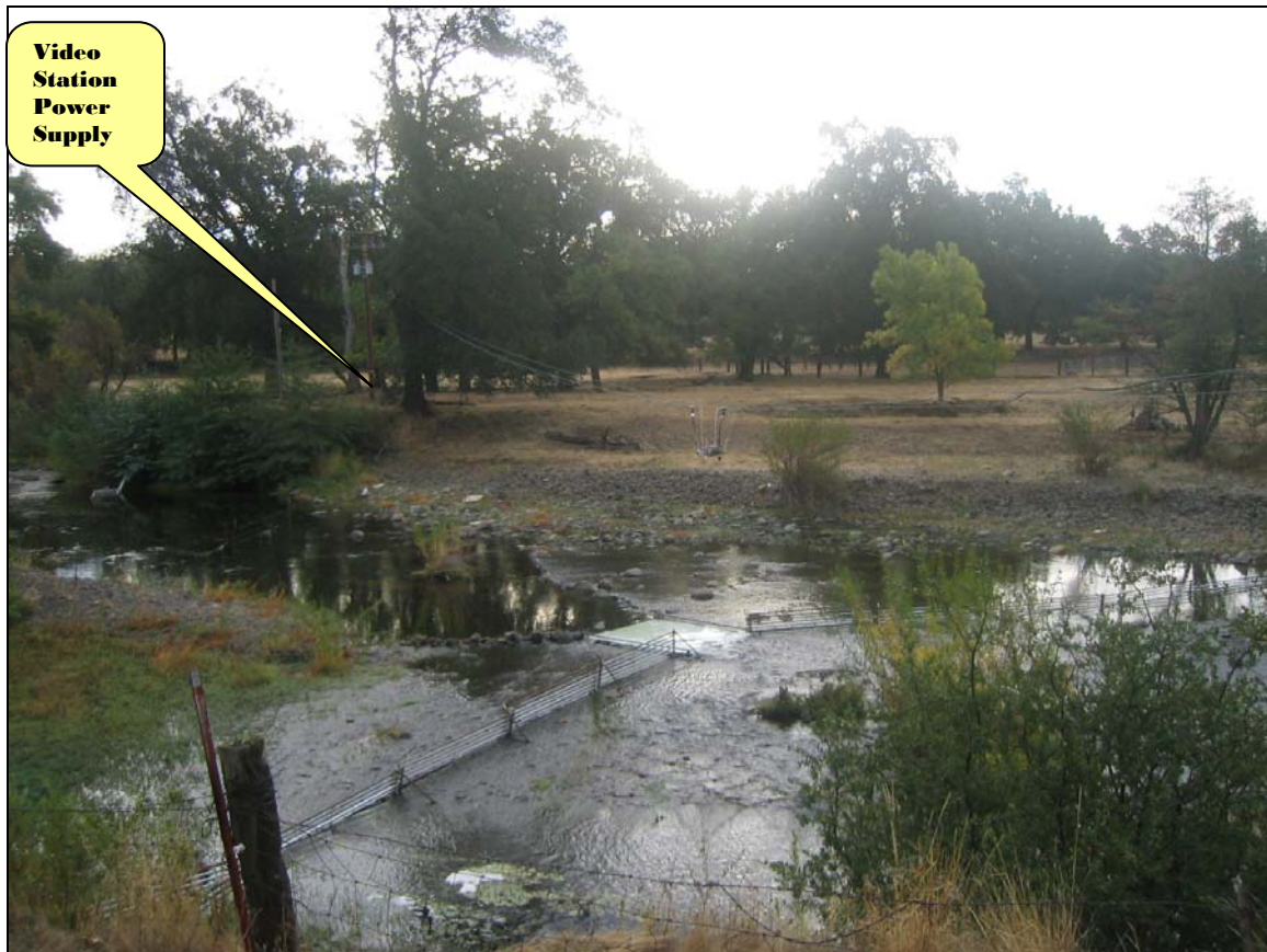
Figure 2. Bear Creek video station power supply box. An active box was available to power the station. A 240 to 120 AC volt transformer was installed to provide standard household power to station equipment. Also showing is the two main cables used to suspend the overhead camera. The VCR lock box is located to the right (not shown).
