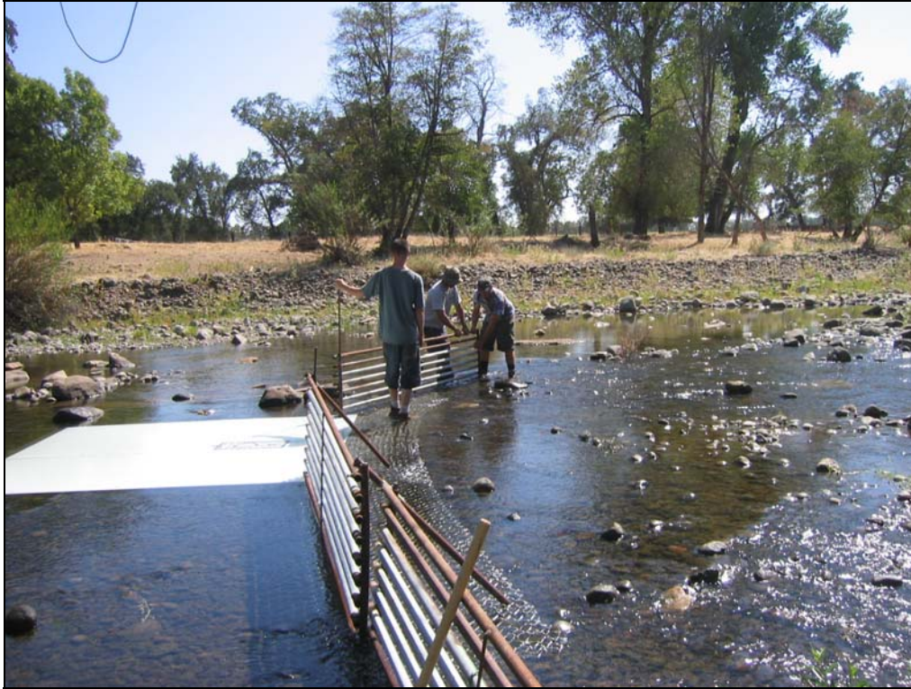
Figure 7. The Bear Creek partial weir showing: the construction of the weir, including the white high density polyethylene (HDPE) sheets staked to the creek bottom to make the observation of passing salmon easier.
